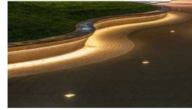
Lighting under bench
